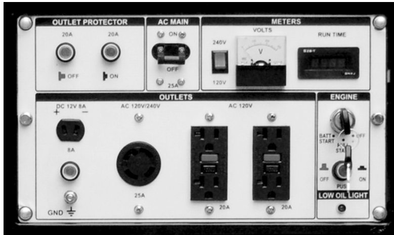
Figure 8 - Outlets Available on this Generator, from left to right, 12V DC, 240/120 AC (NEMA L14-30 plug) and 120V AC
