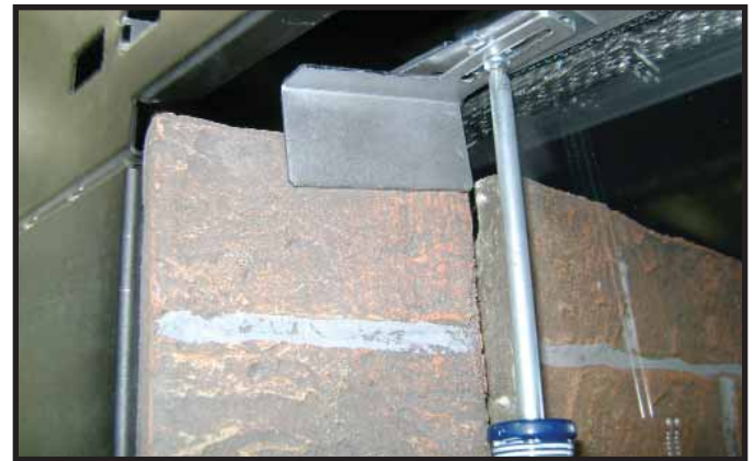
Figure 14.26 Side Refractory Brackets
