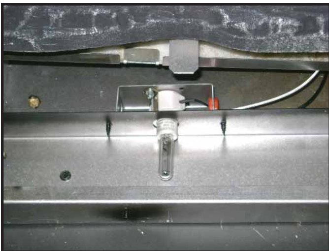
Figure 14.10 Ember Light Bulb Installed
