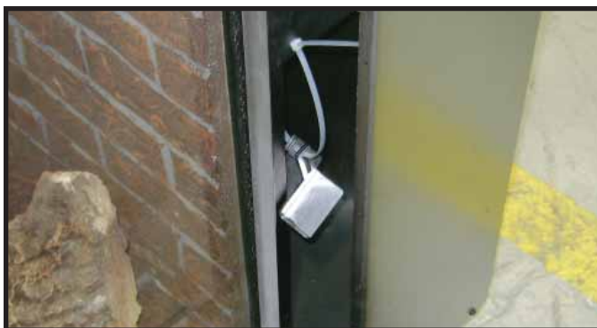
Figure 14.24 Shipping Location of Refractory Brackets
